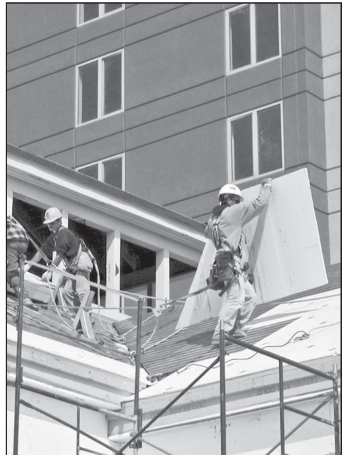
McShane Construction Company employees work on the Hilton Garden Inn-O'Hare in Des Plaines, which opened in the summer of 2005. McShane is one of 20 Builders Association members enhancing the safety of its jobsites by taking part in the OSHA Partnership. Photo provided.
